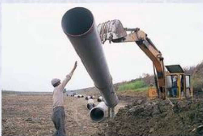
▲ 農田灌溉工程 Irrigation engineering
