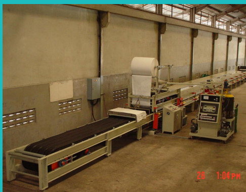
Bridge-Type PU Sandwich-Board Production Line
